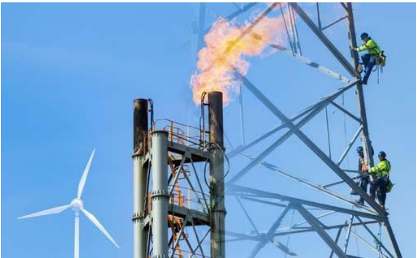
National Grid gas distribution operations
